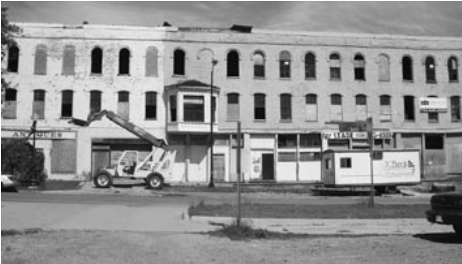
The Thompson Building at the corner of River and Cross Streets was once used to manufacture toys, pull wagons, scooters, and farm implements. It is currently being renovated.
