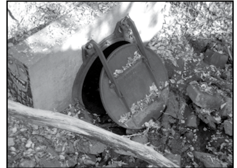
The opening is approximately three feet high and has a partially closed hinged cover
