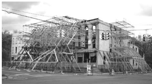
The shell of the Thompson Block building is now being supported by bracing until it can be determined if the façade can be saved.
