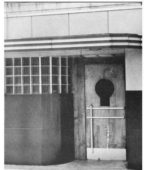
The shape of the keyhole door has changed from the original design and a mail slot has been added.
