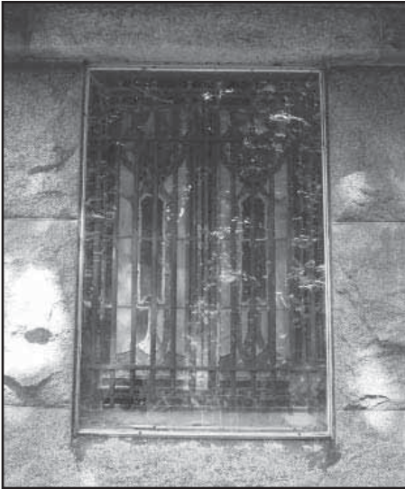
At the rear of the mausoleum is a stained glass window that is protected by a wrought iron grill and a sheet of clear plastic
